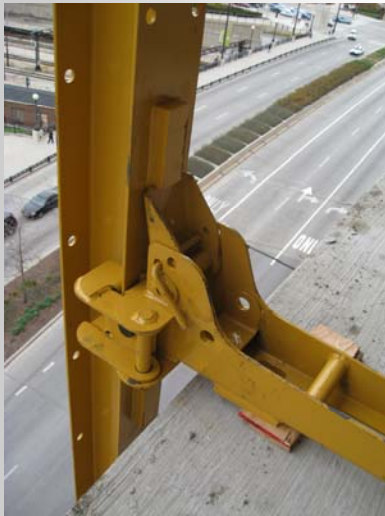
Edge of slab to lifting beam distance substantially reduced (Note: Shoe and lifting beam assembly shown during installation without exterior panel.)
